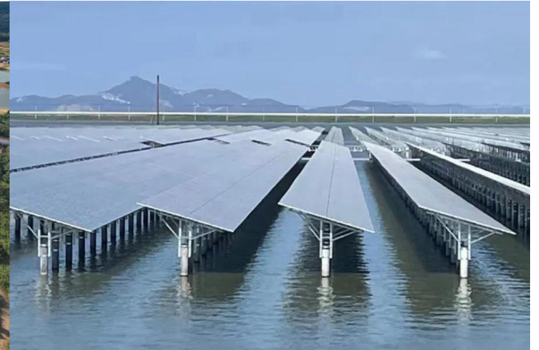
Fishery Power Plant
