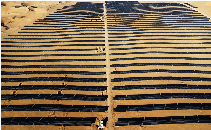
Desert Power Plant
